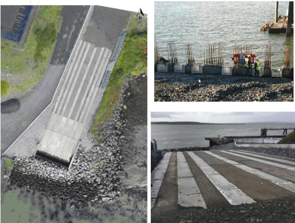
Figure 4.27: Concrete ‘slipway’ structure at Moneypoint. A similar landfall design is proposed for the 400 kV cable landfall works. Aerial view (left), cable trough installation (top right) and top surface (bottom right)
