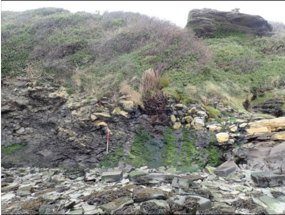
Figure 11.12: North-facing view of upper foreshore and cliff face at centreline of proposed northern landfall (1m scale)
